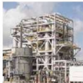
Step 3: Gas clean up and syngas heat recovery (to generate renewable power)
